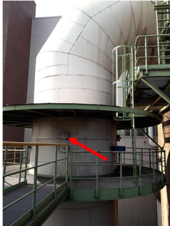
Figure 2: Installation flange in a gas duct
