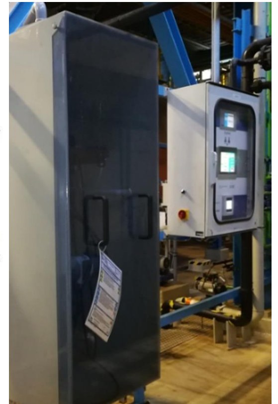
At Outokumpu strip pickling line
